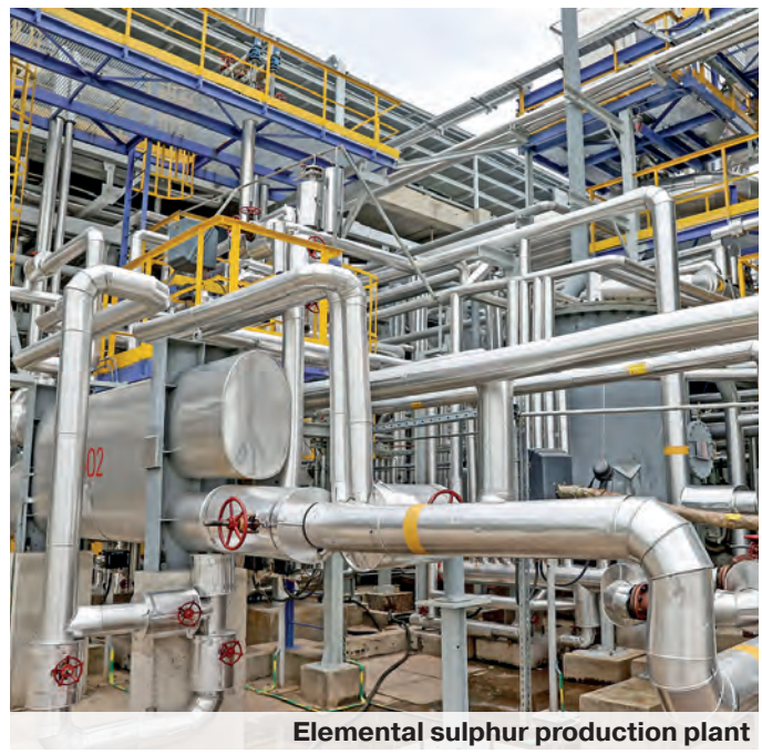
Elemental sulphur production plant
