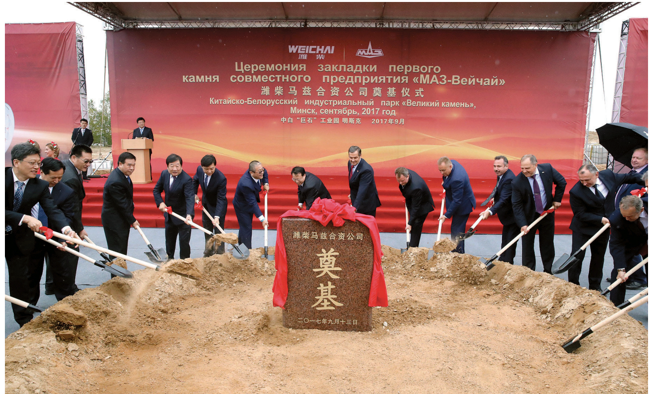
During the first stone laying ceremony on the construction site of MAZ-Weichai
