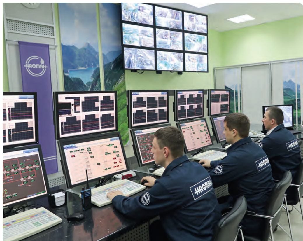
Control over operation of all systems conducted at main dispatching office
