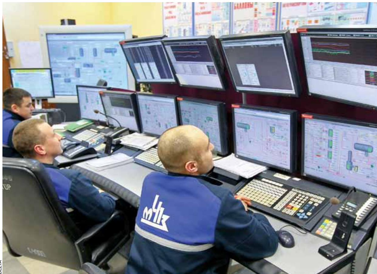
Technological process is under control at Mozyr Oil Refinery
