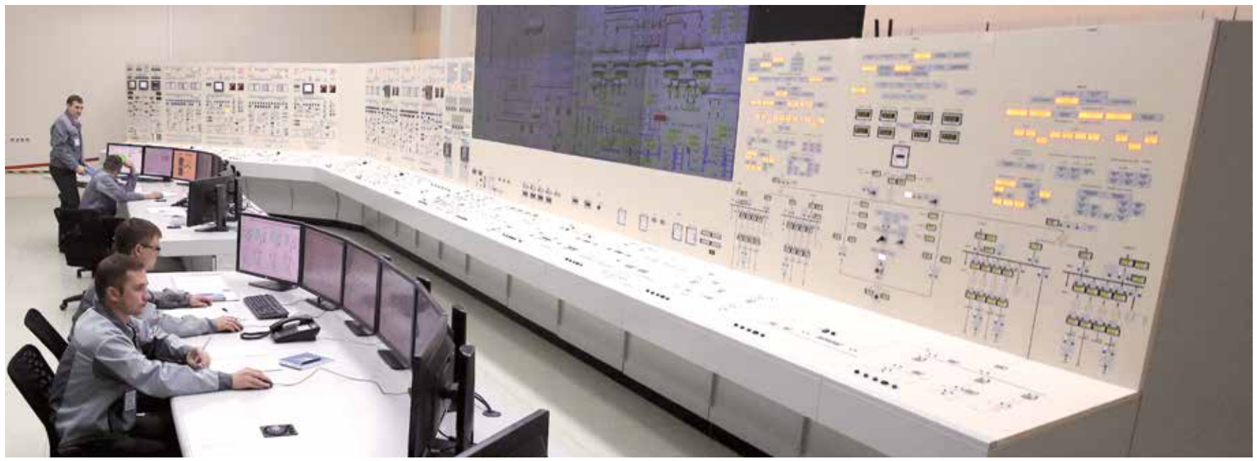
Control board of energy unit at Belarusian nuclear power station
