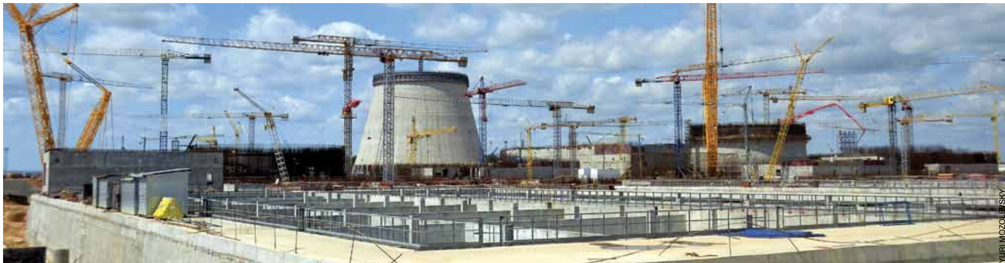
Construction of the Belarusian nuclear power station in line with strict schedule
